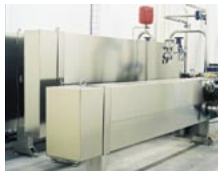
Heat exchanger sludge/water and heat exchanger unit sludge/sludge from Läckeby Products installed in Älmhult, Sweden.
