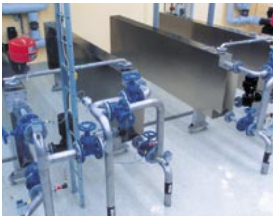
Two heat exchanger units sludge/sludge installed at Vimmerby wastewater treatment works in Sweden.
